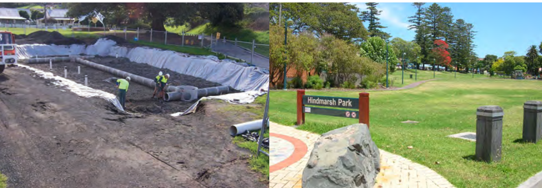
HydroCon pipe system at Hindmarsh Park, Kiama - stormwater harvesting and reuse during and after installation.
