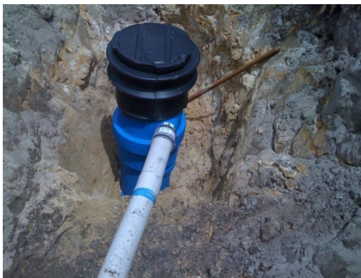
Figure 5 Outlet pipe from HF400 unit to Versitank storage chamber
