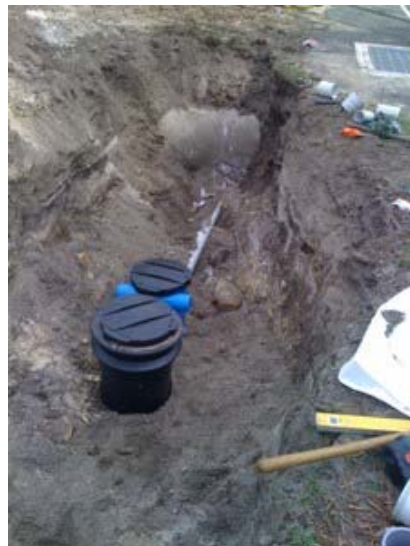
Figure 4 HF400 unit and silt trap attached to underside of 675 mm diameter stormwater pipe
